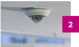
7 Fire alarm and voice evacuation
